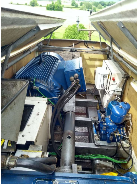
View inside Nacelle.
